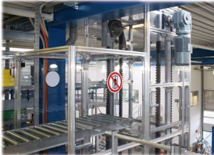
▼ Discharge station of a Portal Lift PH253.
